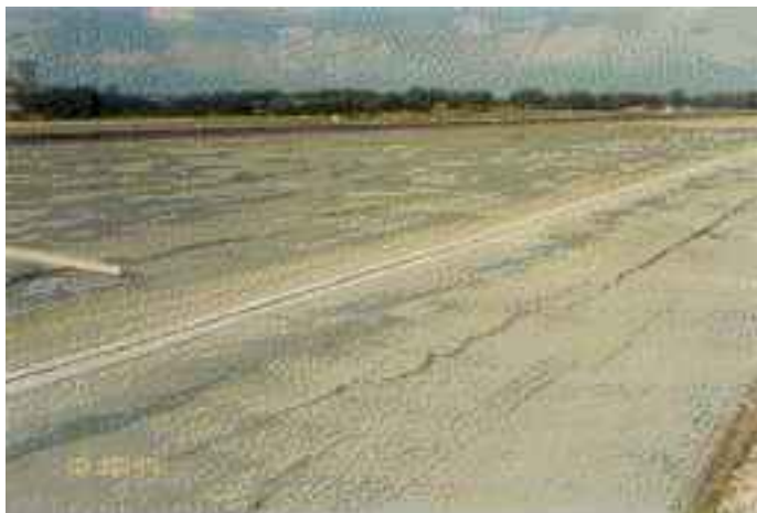
Figure 1 Severe longitudinal cracking and differential settlement and heaving taking place on the surface of a pavement based on an expansive clayey subgrade
