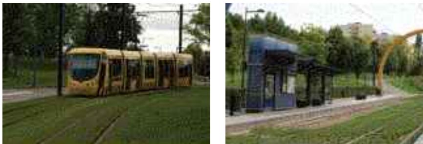
Figure 5 Perfect green track (left) in Mulhouse and the damaged green track at a terminal stop (right) caused by (too) long idle time and multiple mechanical impacts by trespassing passengers
