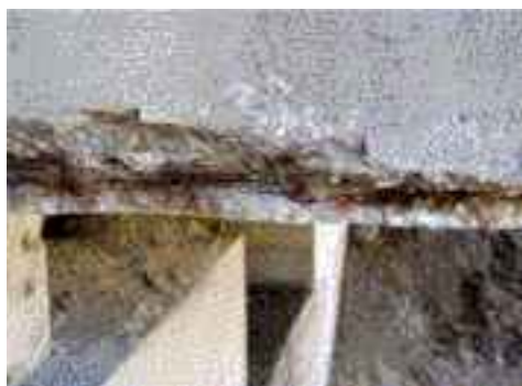
Figure 3 Exposed, corroded reinforcement
