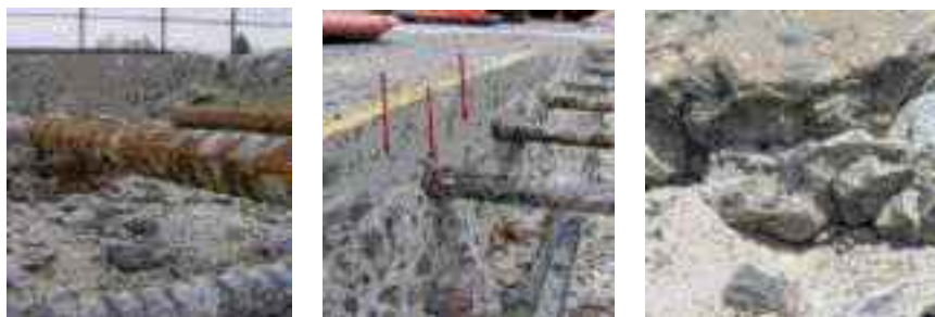
Figure 1 Rebar corrosion, delamination and concrete degradation.
