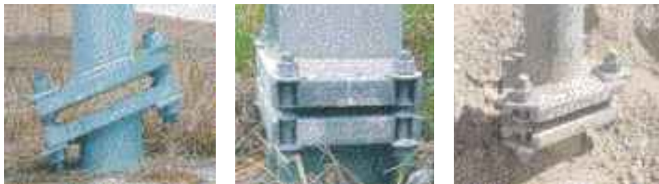
Figure 14 Examples of the break-away NE columns [4]
