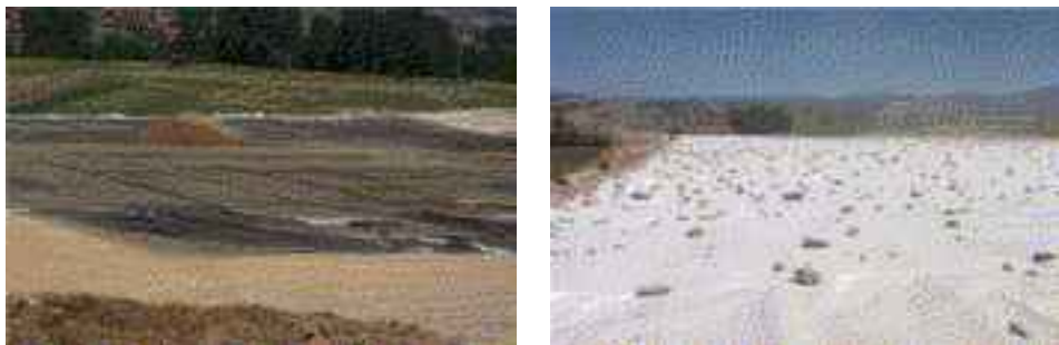
Figure 9 The geogrids were placed over the full embankment width, starting at app. 373 m altitude, which is approx. 0.5 m above the 100–year flood level. A combigrid was installed underneath the road base course over a width of approx 30.9 m. A combigrid was installed transversely to the road axis, with an overlapping of a min 300 mm in both adjacent and longitudinal directions.
