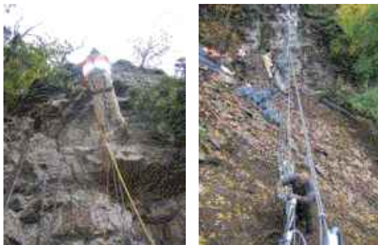
Figure 5 Drilling being carried out on ropes (left) and fixing of the ring net after the installation of support ropes (right).
