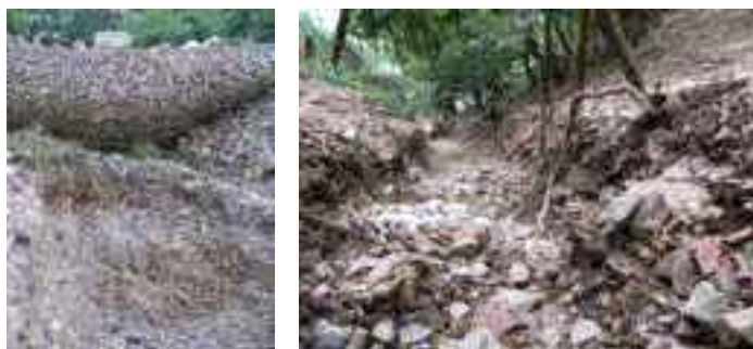
Figure 2 Installed ring net barrier of 2005 filled after the event in July 2008 (left) and gully after the same event (right).
