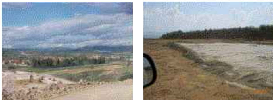
Figure 6 View of the beginning of embankment construction with material from cutting, which was to be used as material category C, and a view of the test field where it was confirmed that this material is not to be placed in the embankment without improvement.
