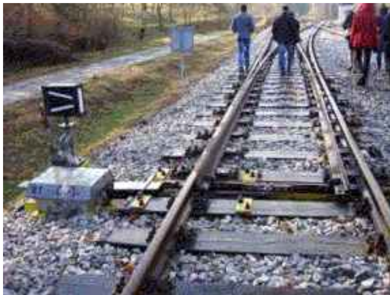
Figure 3 Disconnector switch on special track
