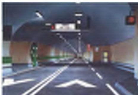
Figure 2 Example of properly installed traffic signs in a tunnel [3]
