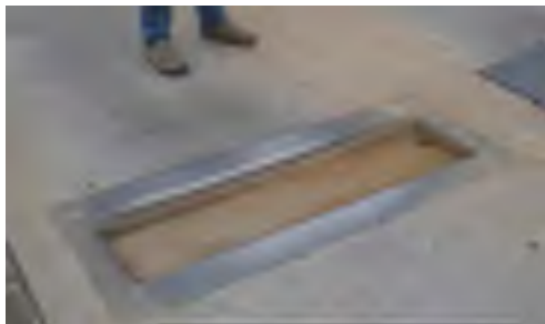
Figure 5 Detail of the pothole track
