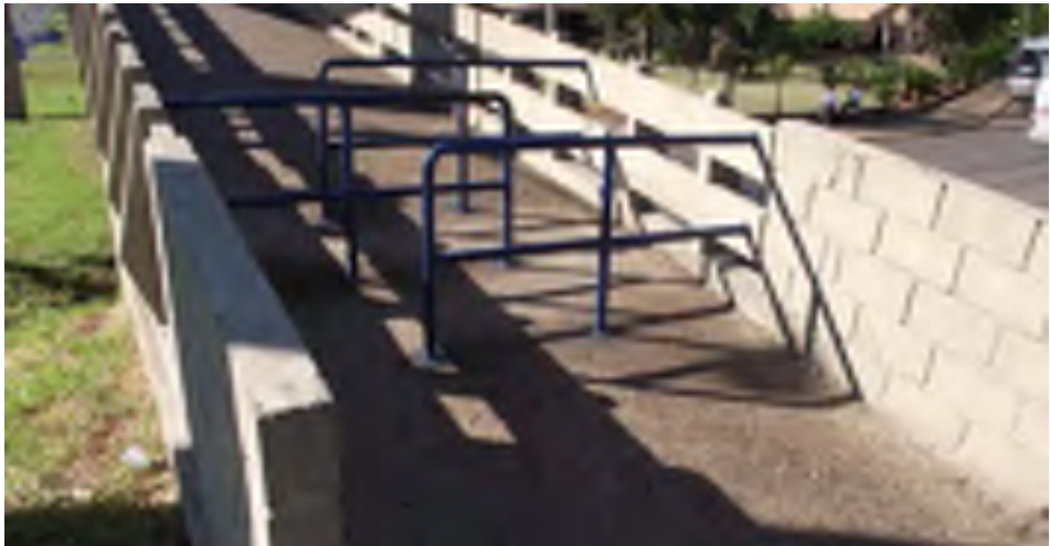
Figure 5 Obstruction in a walkway giving access to a stopping point located on Zeferino Vaz highway, shown in Figure 6
