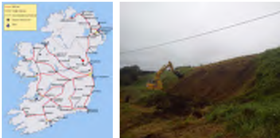
Figure 7 a) Location of embankment shown by red dot, b) photo of embankment preparation for instrumentation
