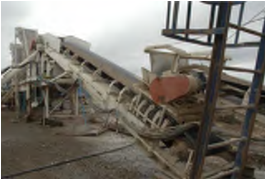
Figure 2 Plant for production of Recyvia® in the bypass of Troyes (France)
