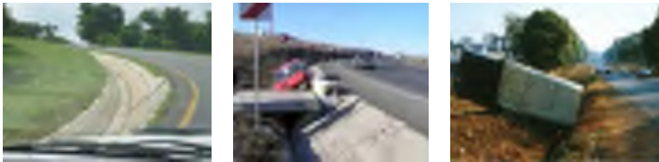
Figure 3 Unsafe drainage structures
