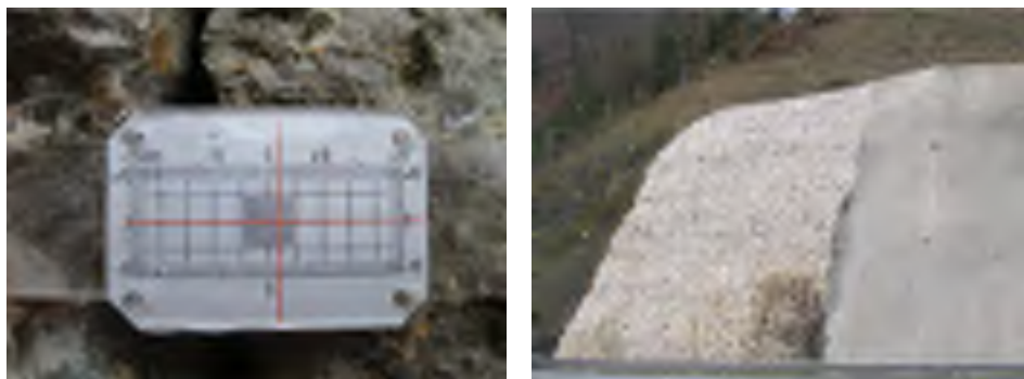
Figure 3 Gornji Macelj 4 – installed crackmeter and vertical crack on the slope
