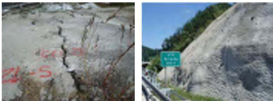
Figure 2 Defects and crack on Straža jug cut
