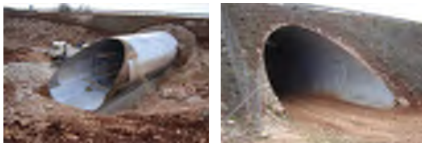
Figure 9 Installation of animal underpass – phase II and animal underpass in km 5+030,00 of Adriatic Highway – ISTRIAN “Y”
