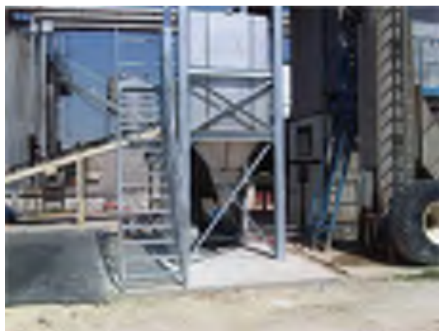
Figure 2 Automated feeding of the additive (Plant CIFA Mityr-Mory, France)
