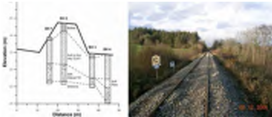
Figure 4 a) Boreholes taken across failure, b) Photo of Enniscorthy Embankment
