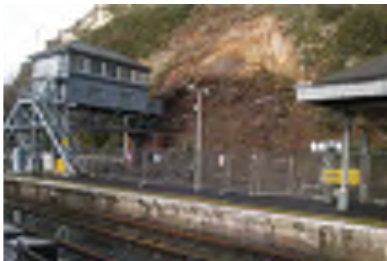
Figure 4 The effects of slope failure of 31/12/2013 on Waterford rail station
