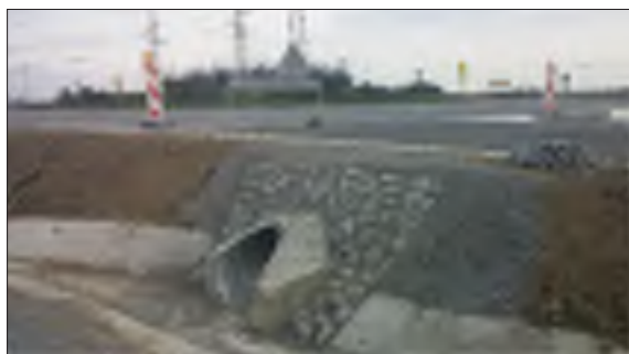
Figure 8 Completed culvert at roundabout entrance (first phase of construction) during construction work
