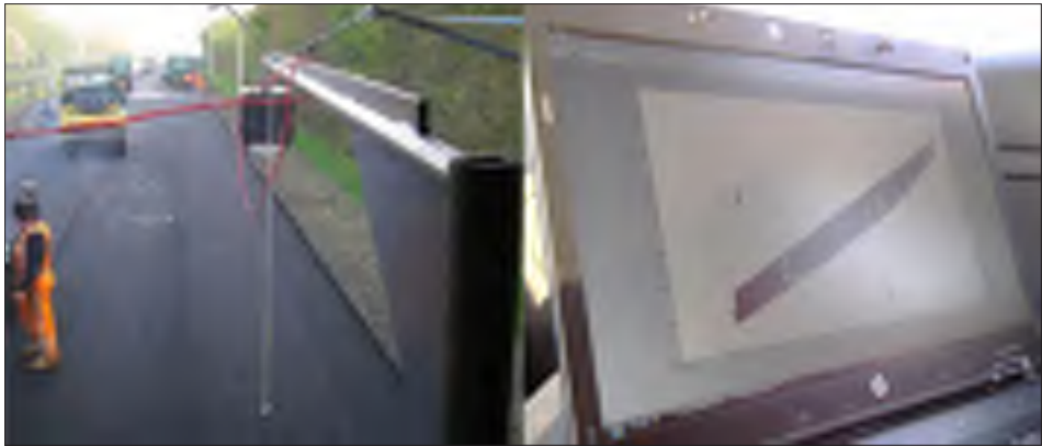
Figure 5 On site temperature measurement with an industrial temperature line scanner (left) and on-site information provision to site management staff during ongoing operations (right)
