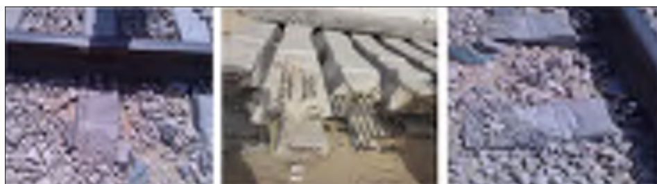
Figure 1 Cracked and Corroded Concrete Sleepers (km 19, 25, 31 & 37)
