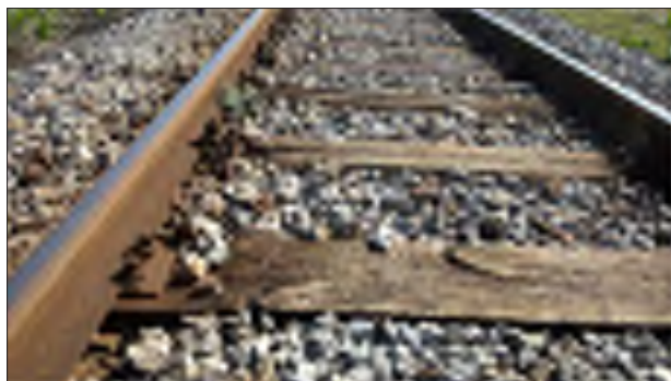
Figure 1 Condition of track type 1
