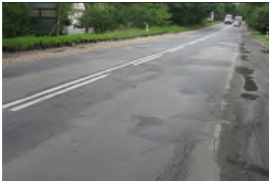
Figure 2 View of damaged pavement on national road 44
