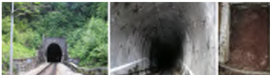
Figure 3 Entrance portal of the tunnel Resnjak, interior of the tunnel and the niche from which the material is falling
