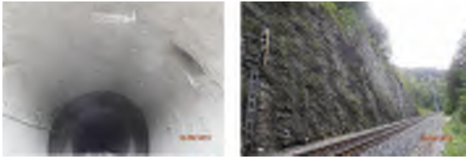
Figure 4 Reconstructed vault of the tunnel Tičevo and cutting exit of the tunnel
