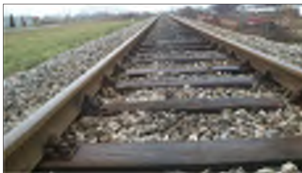
Figure 2 Condition of track type 2
