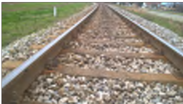
Figure 5 Condition of track type 4
