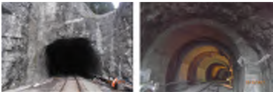
Figure 5 Cutting approach and entrance portal of the tunnel Kloštar and the rings at the exit part of the tunnel after reconstruction
