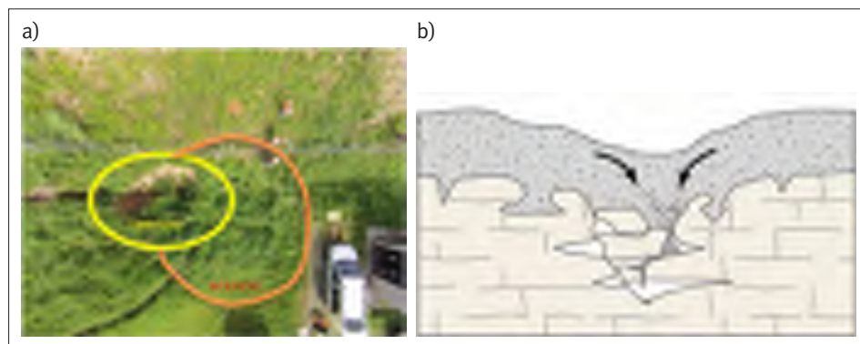
Figure 5 Suffusion sinkhole in 46 th km: a) location, b) suffusion mechanism [7]
