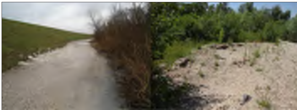
Figure 1 Seepage through an levee and foundation soil
