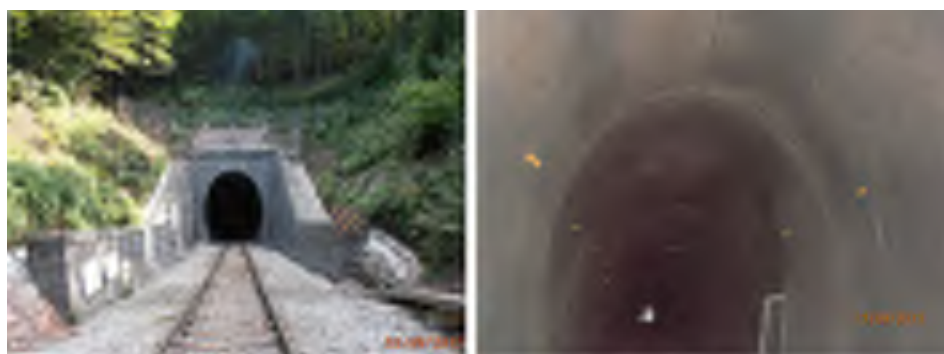
Figure 6 Cutting exit of tunnel Resnjak and interior of the tunnel after reconstruction
