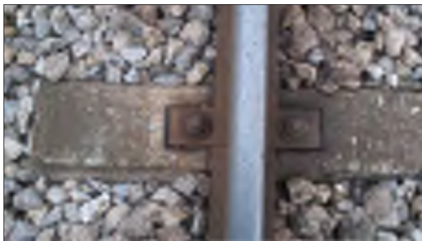
Figure 3 Condition of track type 3
